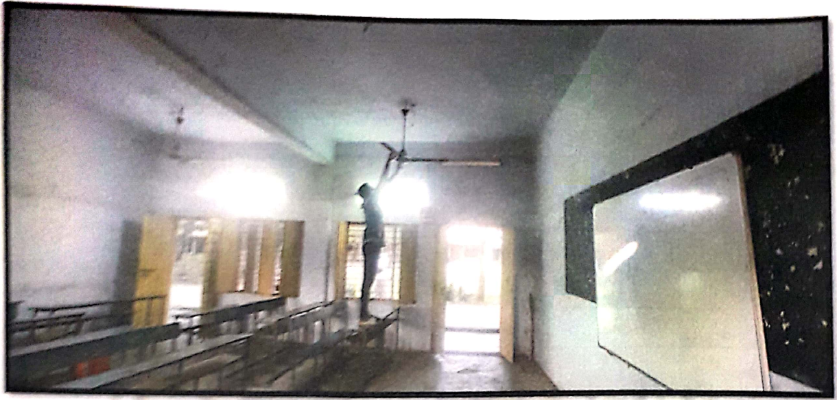
Repairing Fans and Arranging New tube lights on 16/09/2023 in B.Sc III (MPCs)
